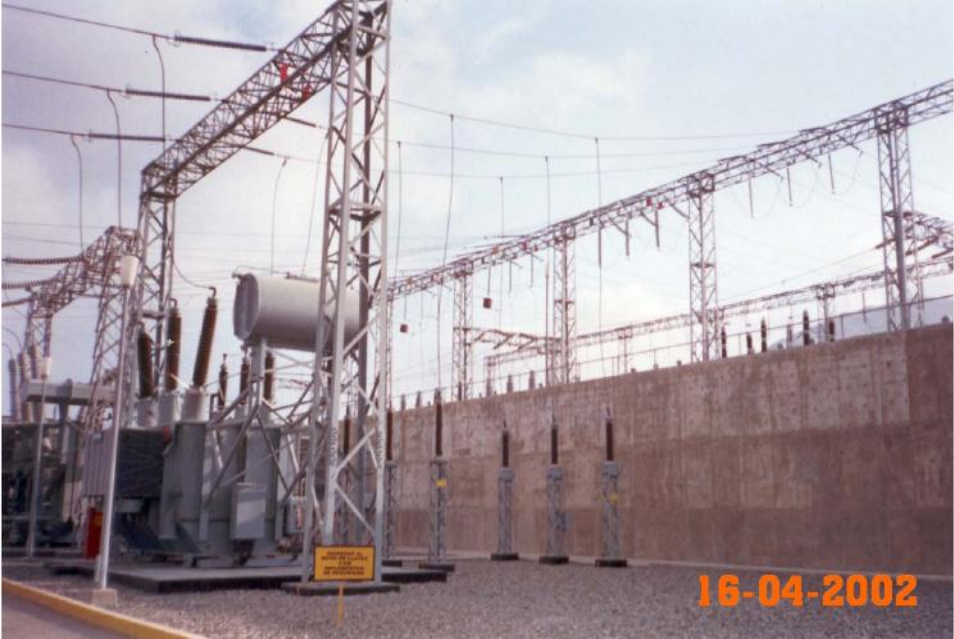
SET CHIMBOTE N° 1 (REP) Auto transformador 220/138/13.8 kV, DE EGENOR, CHIMBOTE – SANTA - ANCASH.
